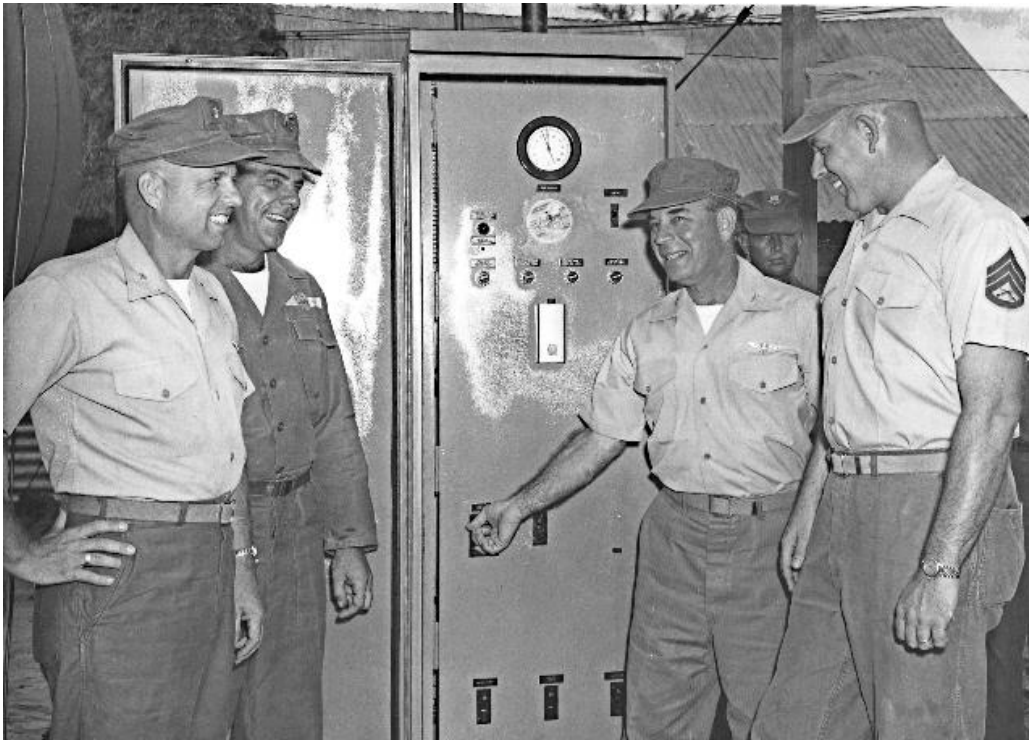
Shufly C.O. Col. Andre Gomez throws the switch activating Shufly's new well pump with SSgt. Karl Nichol, MABS-16, Sub Unit # 2 utilities chief by his side, as Sub Unit commanding officer, Lt. Col. Earl Cassidy far left and Seabee crew boss, EO1 Pete Welty look on.
